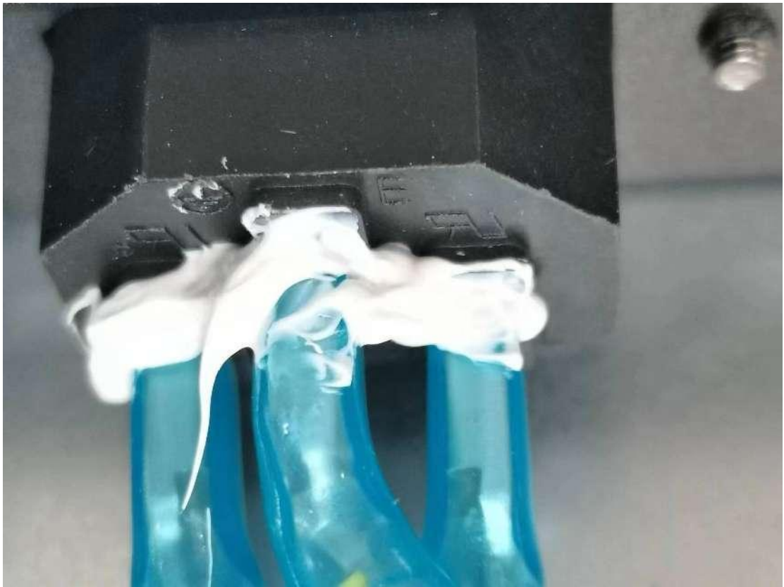
Figure 16. Earthing terminal view
