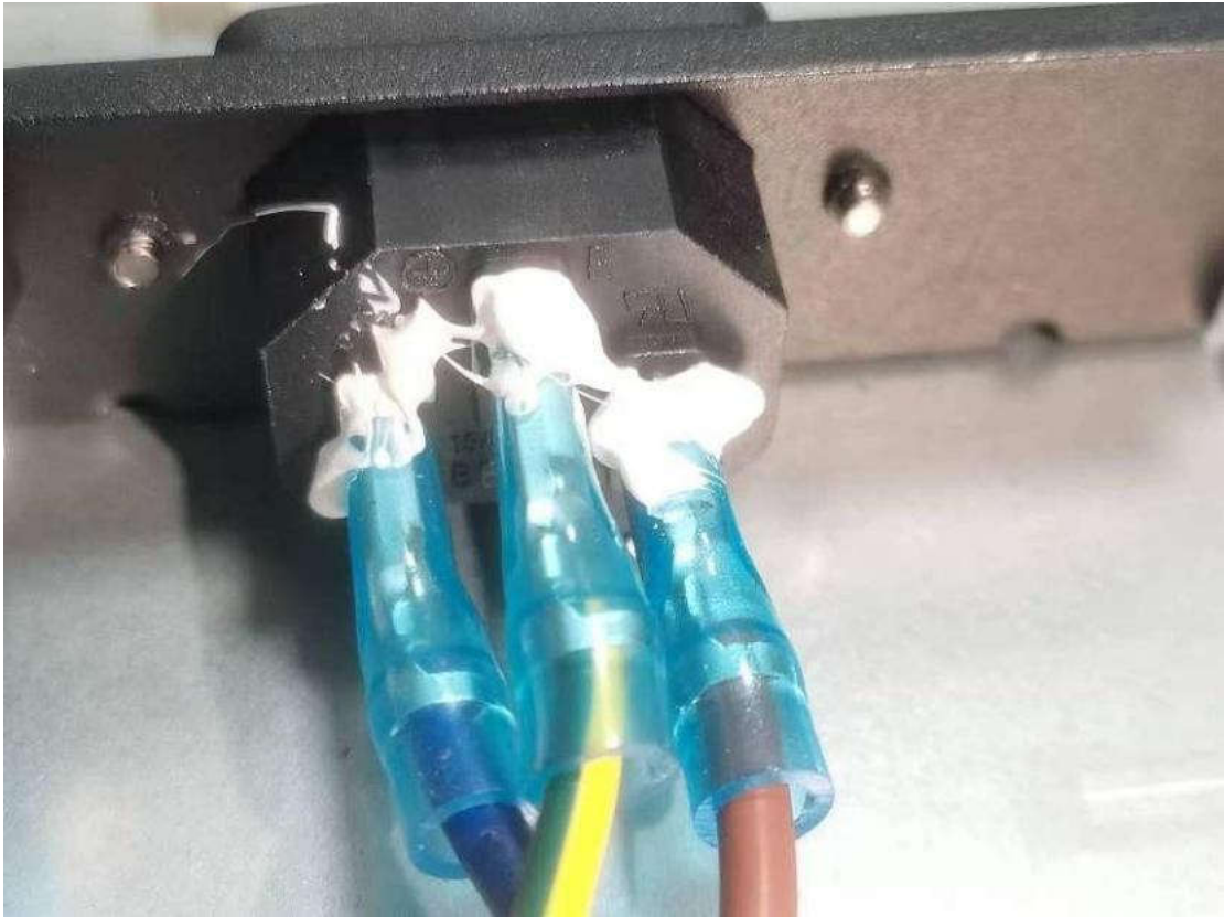
Figure 16. Earthing terminal view
