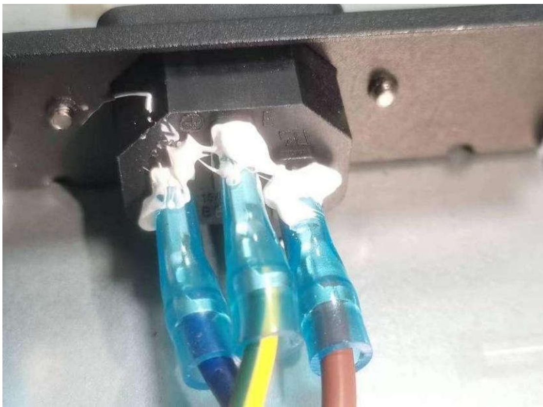
Figure 16. Earthing terminal view
