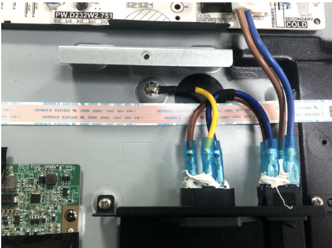
Figure 17. Bonding terminal view
